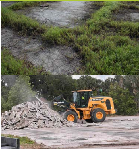
Concrete pads, the bases of the old greenhouses; Photo: Joyce Stefancic. Areas being scraped and pads taken out. Photo: Deborah Green.
