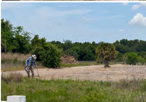
Concrete pads being removed, late April 2026, Photo: Deborah Green. Lance Hart marking which pads to save, Photo: Jack Horton.
