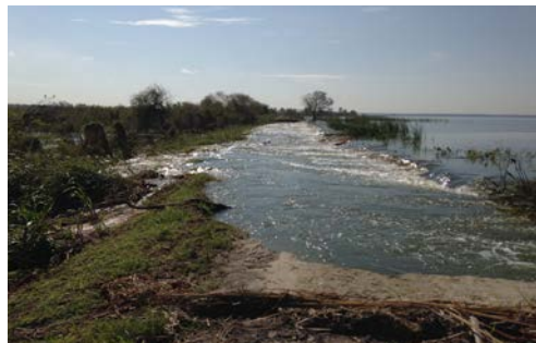
Breach in farm levee south of the Lake Apopka North Shore historic pumphouse. Photo: Deborah Green
